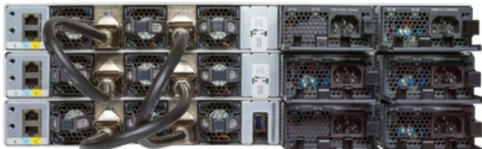
Figure 5. Cisco Catalyst 9300 Series switch stack units
