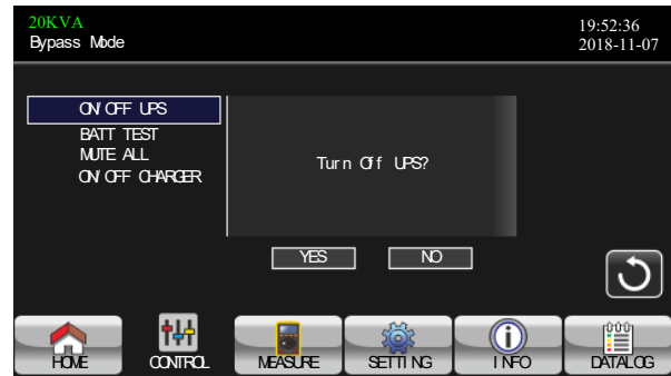
TURN OFF UPS
